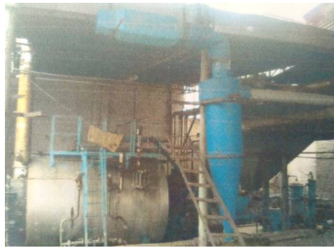
Fig.8 Photo taken during testing of Cyclone Separator
